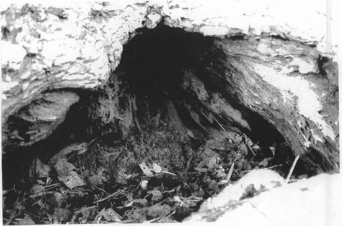
Closeup of cavity at base near sidewalk
