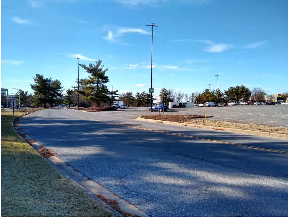
FIGURE 5. Vicinity of Walkers Run as piped under the Lake Forest parking lot.
