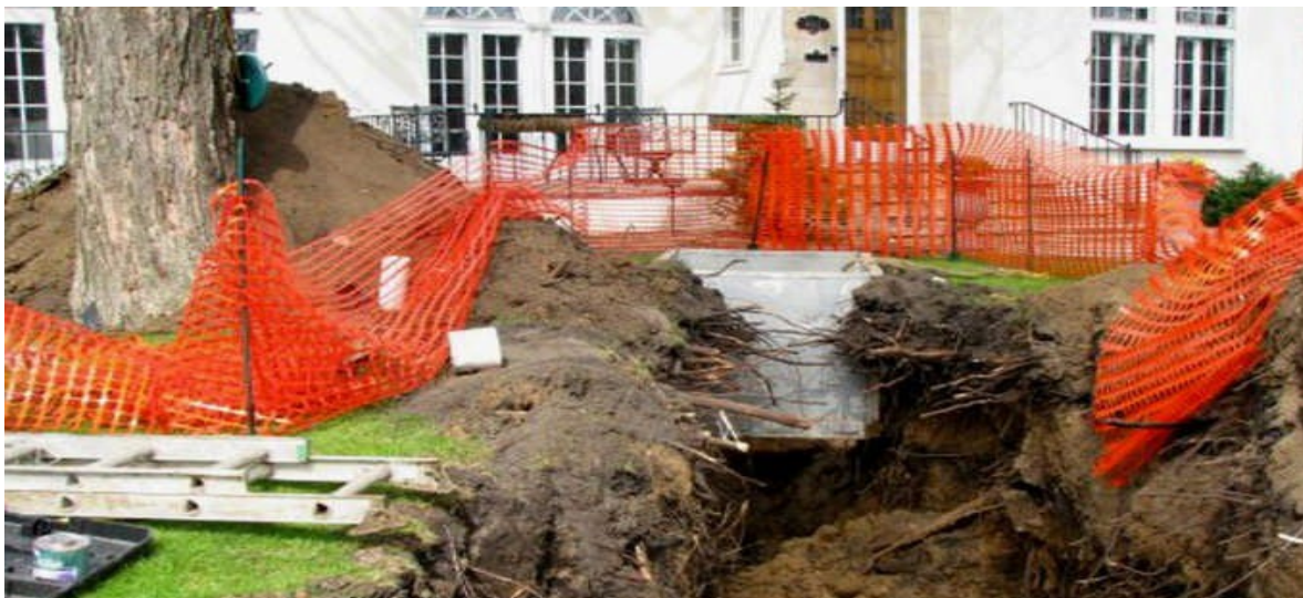
Figure 25: Note that the face of excavation is typically ragged and the roots to be pruned are at varying setbacks. Pruning only required on left side (one payment line) where the live roots exist.
